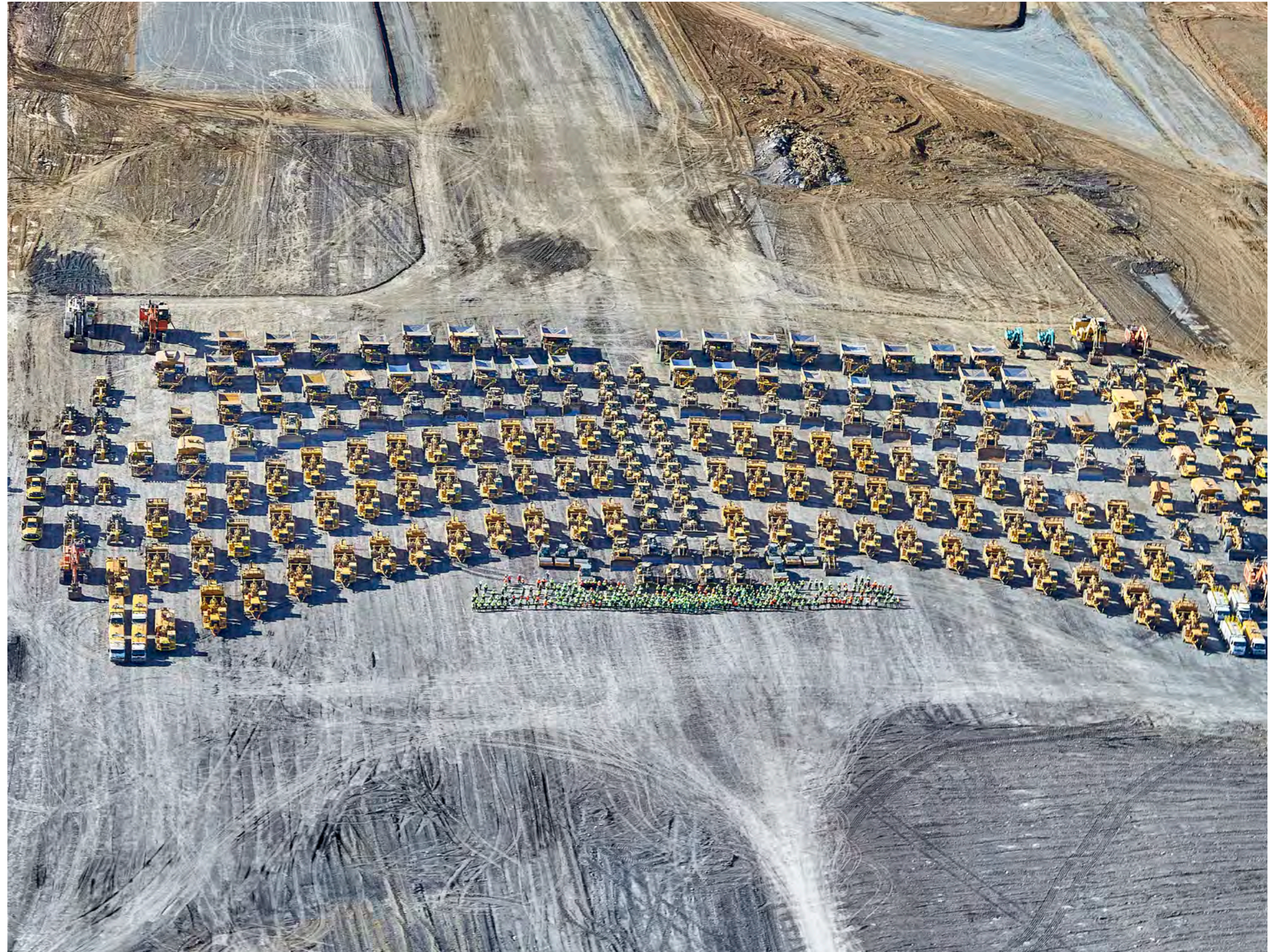
260 pieces of earthmoving equipment helped prepare the site of Sydney's new airport.
