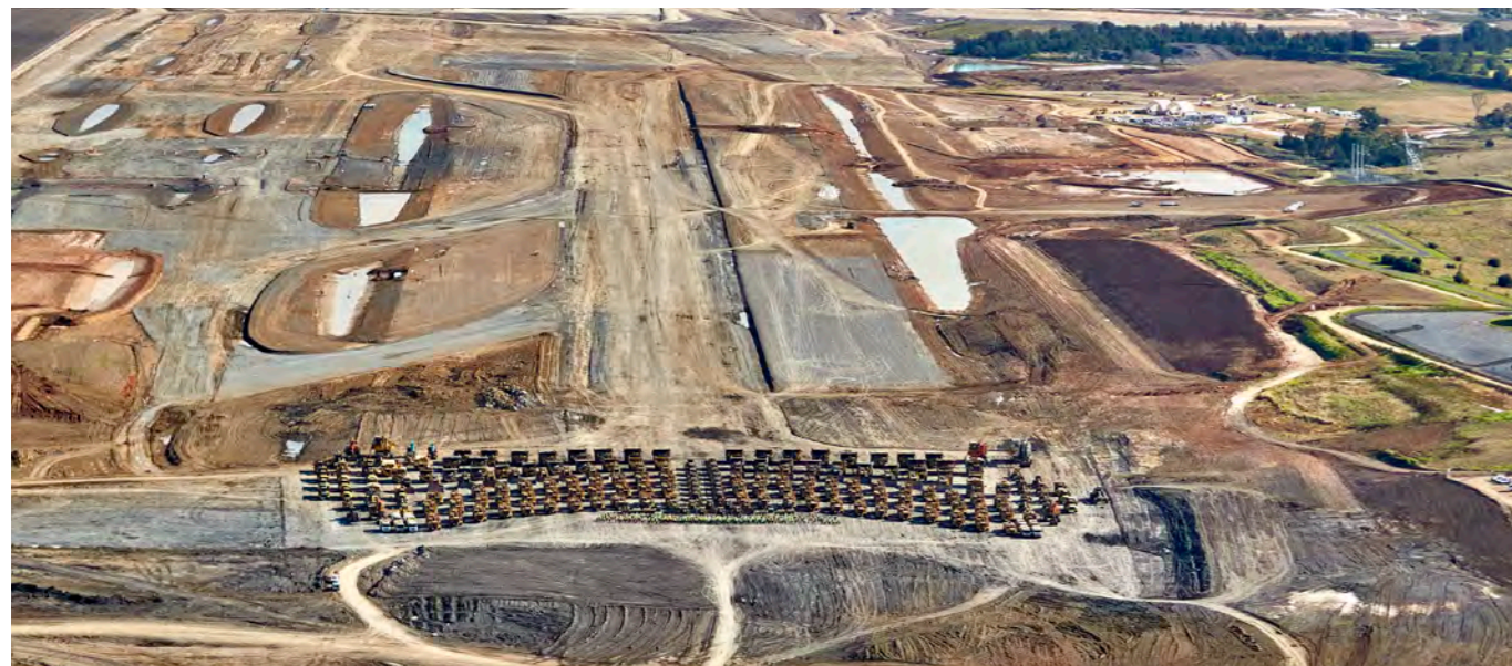
By the end of June 2021, 18 million cubic metres of earth had been moved.
