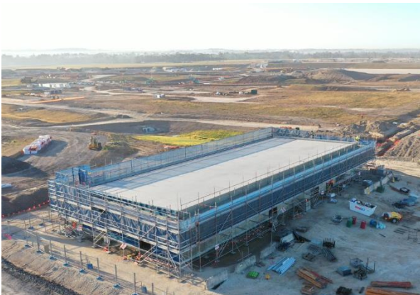
Aerial photo of one of the airfield lighting and equipment rooms, taken June 2023
