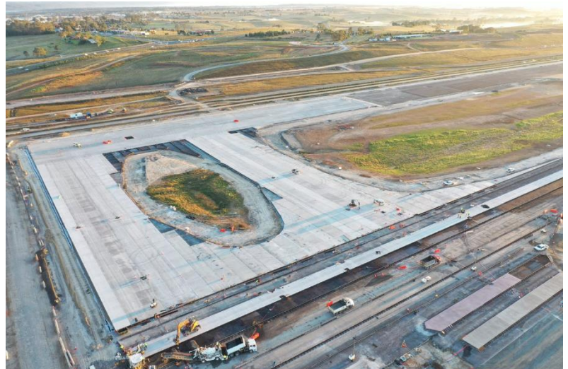
Aerial photo of the concrete pavement on the end of the runway, taken June 2023
