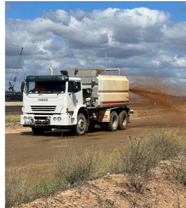
Figure 25 - ACP application of Dustex on haul roads to reduce dust generation. Opposite page: Figure 26 - Reuse of site captured water to reduce dust generation
