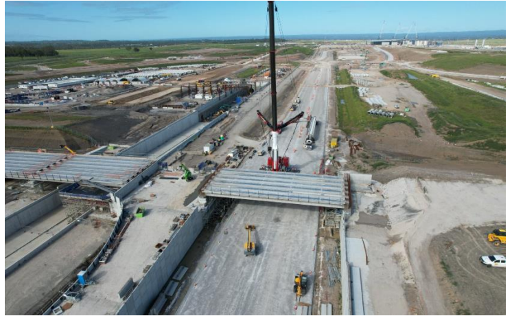
Aerial photo of the bridge connecting the Business Precinct to the internal road network, taken February 2024
