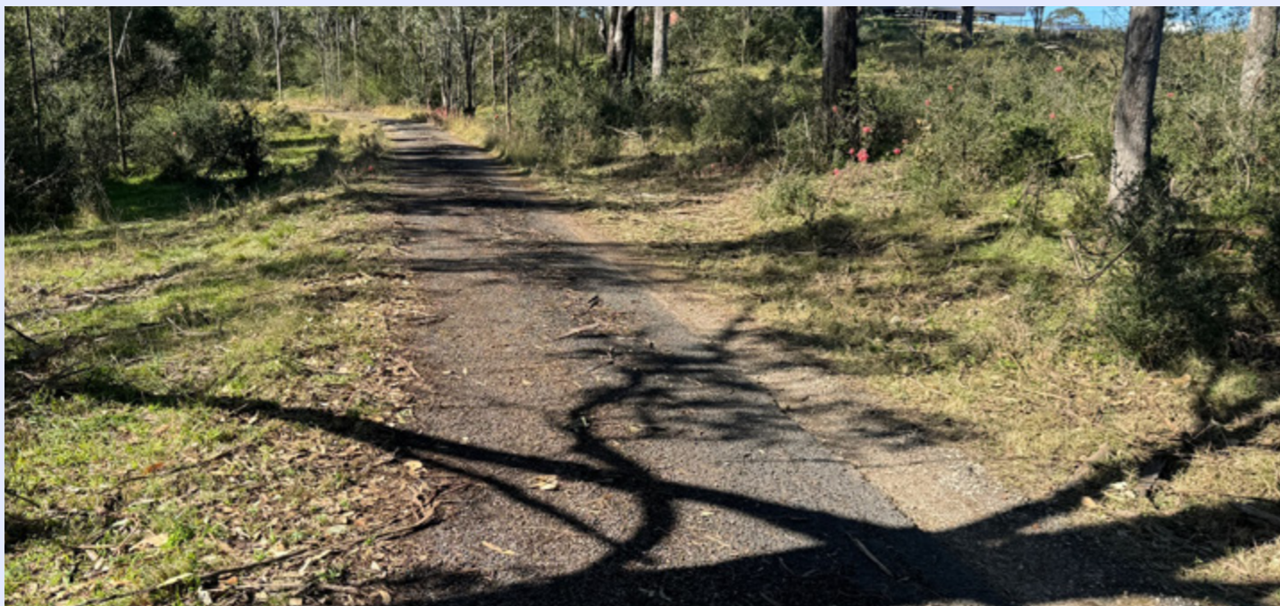
Figure 27 - Comparison following weed removal along Willowdene access track
