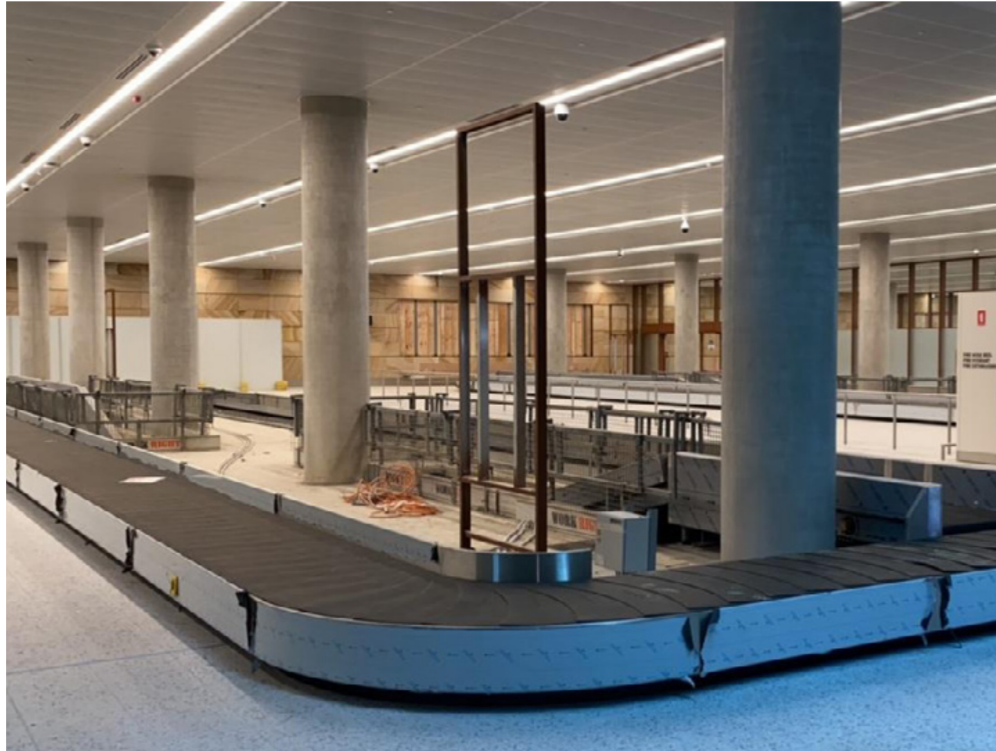
Figure 2 - Baggage Handling System (BHS)
